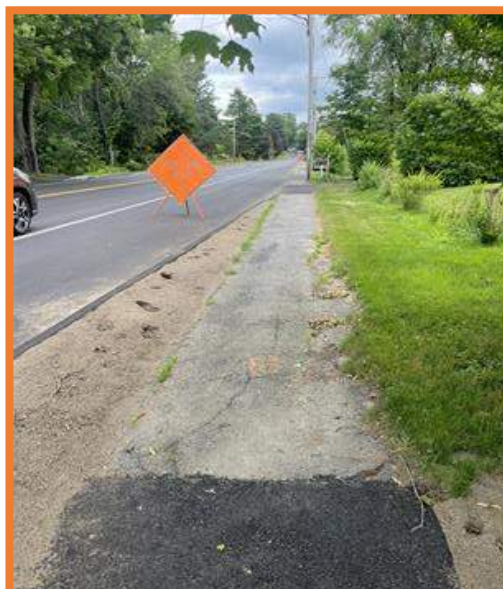
Sidewalk graded at ‘Poor’ (Main Street)
