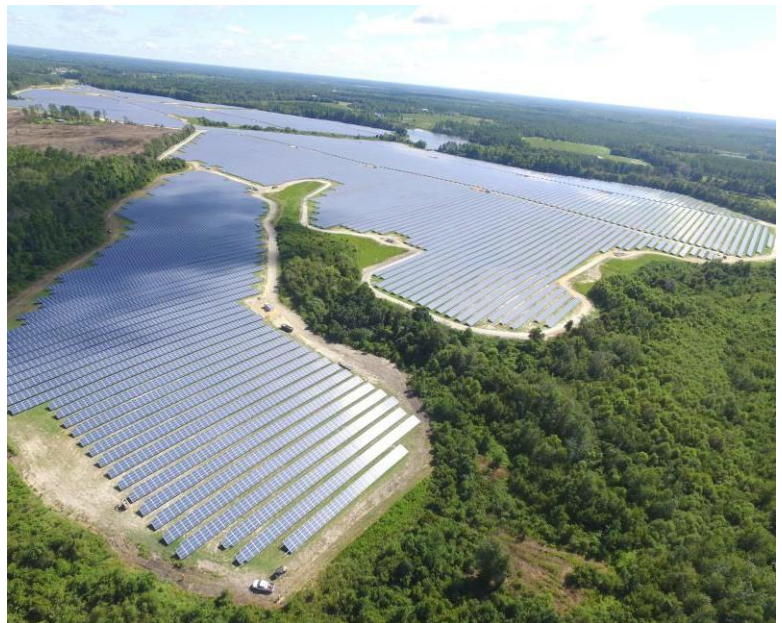
A ground-mounted solar system sited in a rural area.
