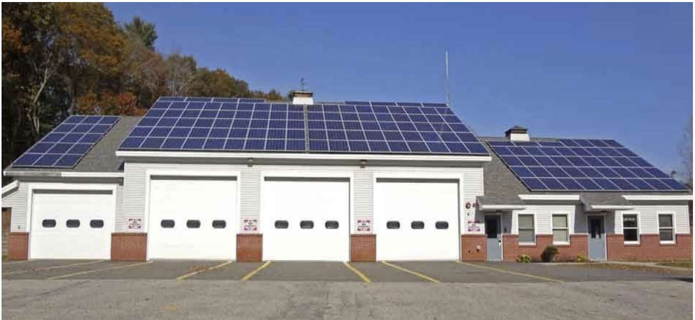
A 40 kW solar electric system installed on the roof of the Windham Fire Department (Photo by ReVision Energy)
