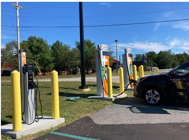
Windham Hannaford ChargePoint Station (Photo by PlugShare)
