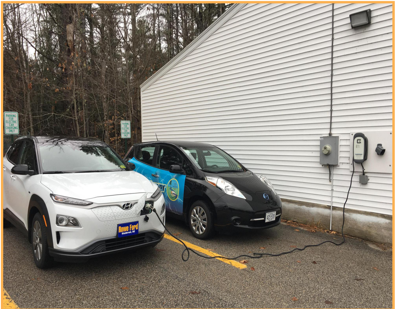
Windham Town Hall EV Charging Station (Photo by PlugShare)
